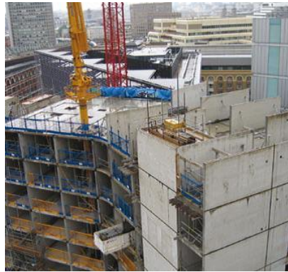
Fig. 3: Hybrid Concrete Construction (Precast twin wall and lattice girder slab with in-situ concrete), Hilton Hotel, Tower Bridge, London [157UK]
