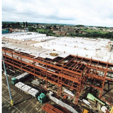
Fig. 5: Mixed Construction (steel frame and precast concrete floor panels) of an industrial building in Ballina, County Mayo [119IRL]
