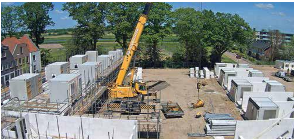
Figure 1. The construction of 18 new homes in the centre of Hardenberg according to the Customised Housing concept.[8]
