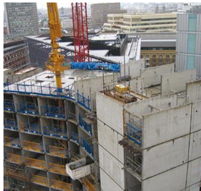
Figure 14. Hybrid Concrete Construction (Precast twin wall and lattice girder slab with in-situ concrete), Hilton Hotel, Tower Bridge, London [68]
